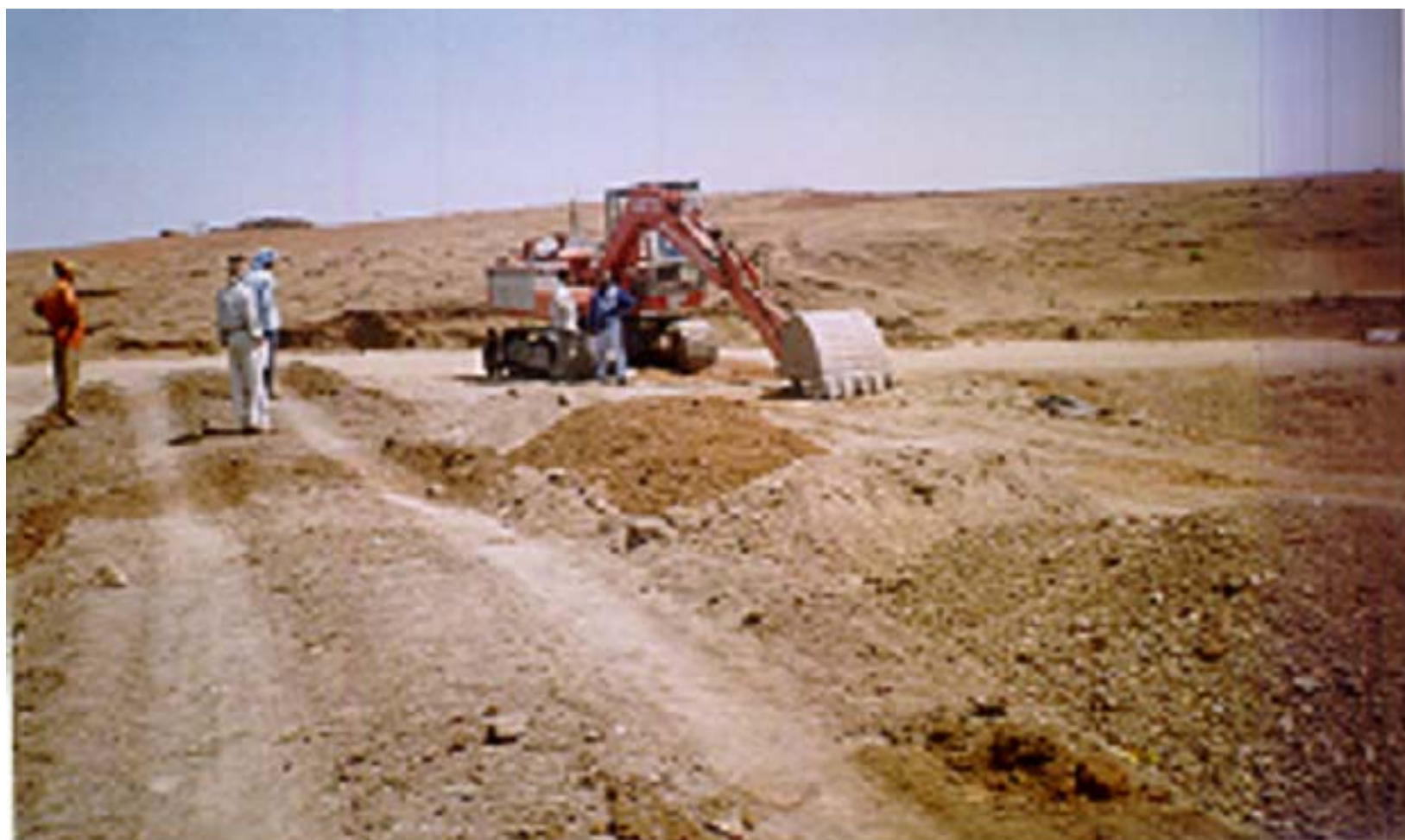
EXCAVATOR IN OPERATION AT RELIEF SITE Village: LANGDI MOHADI, BARWANI DISTT., M.P.
